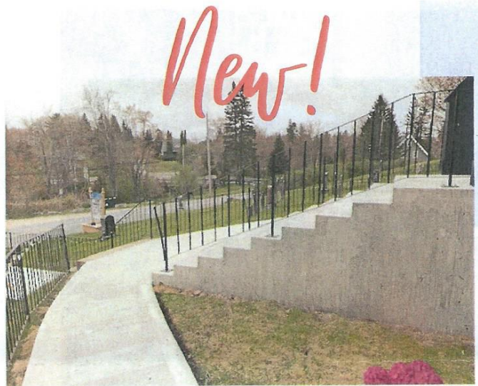
We have great new concrete front steps and walkway thanks in part to assistance from the Shatford trust. The contractor was Steven Hare. New railing by G Veniot Metal. Also included in the photo is the top of a dwarf rhododendron donated and planted in memory of Hilda Duncan.
